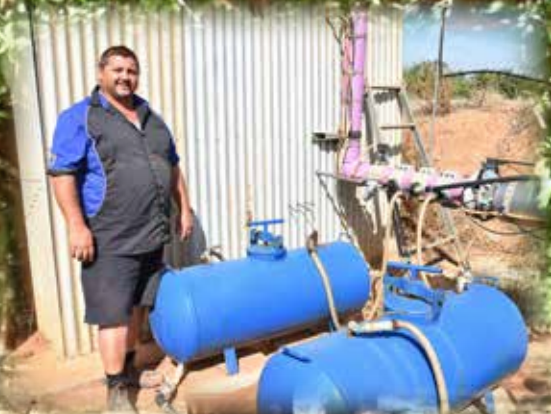
Phillip with some of the irrigation and fertiliser injection infrastructure at the family's Angle Vale orchard.
