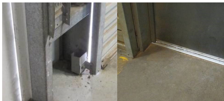
Figure 8: Small holes (>6mm) allow entry into facilities. This is especially important around roller doors where it is difficult to reduce gaps. (a) Small gap alongside roller door allowing entry. (b) Well fitting metal door strips improve management of entry of mice.
